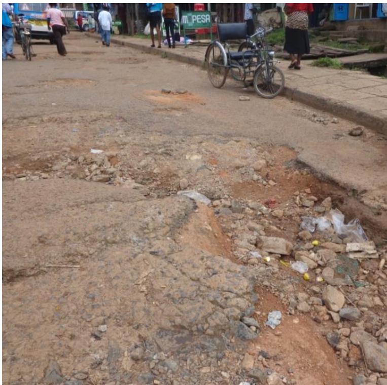
Plate 4.9: Eroded Drop off in Kakamega Terminus
