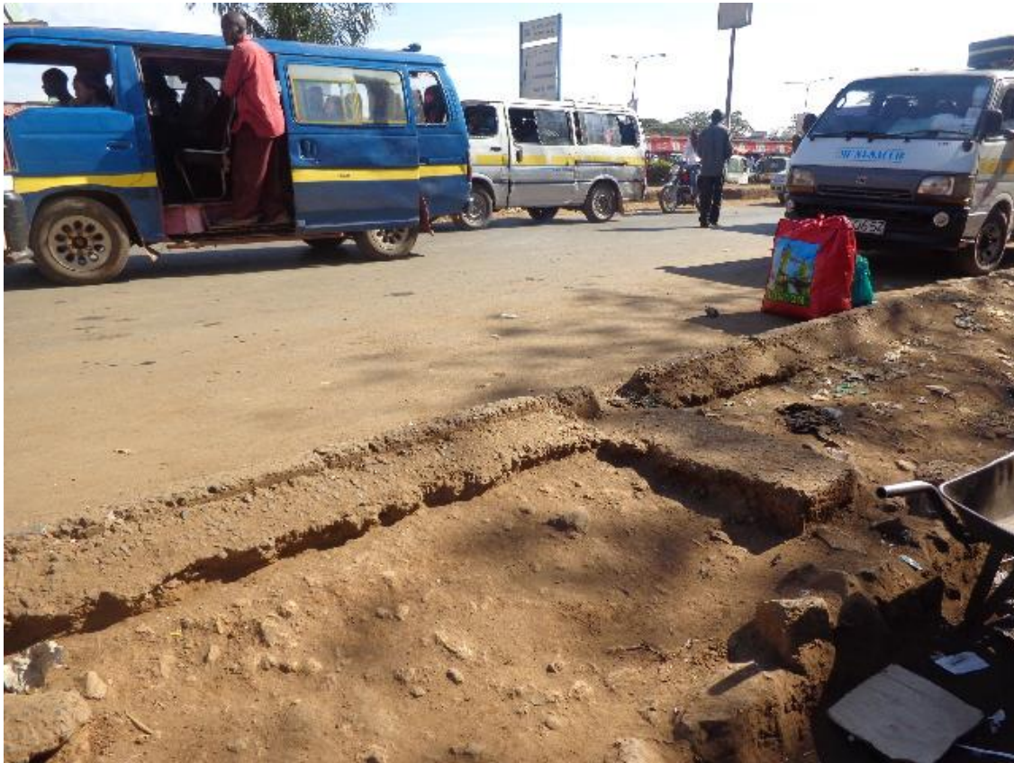
Plate 4.11: Eroded Pavement in Kisumu Bus Terminus
