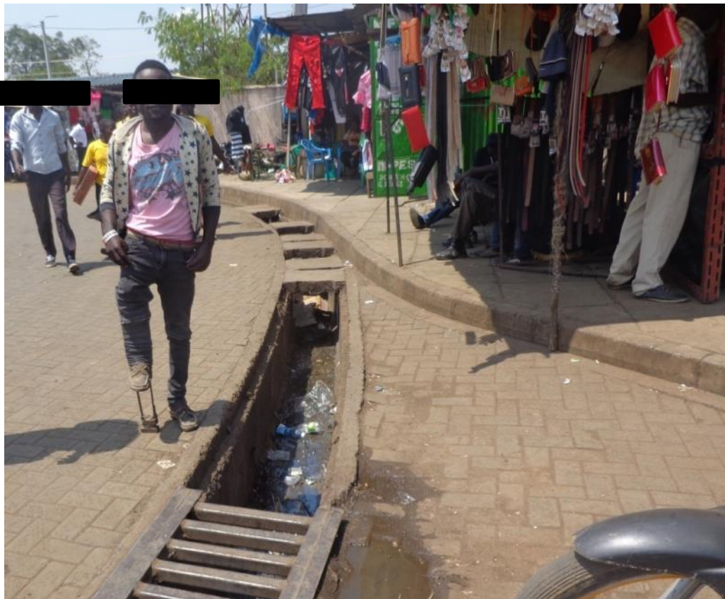
Plate 4.12: Special Boot User Walking Along Area Having Missing Slabs
