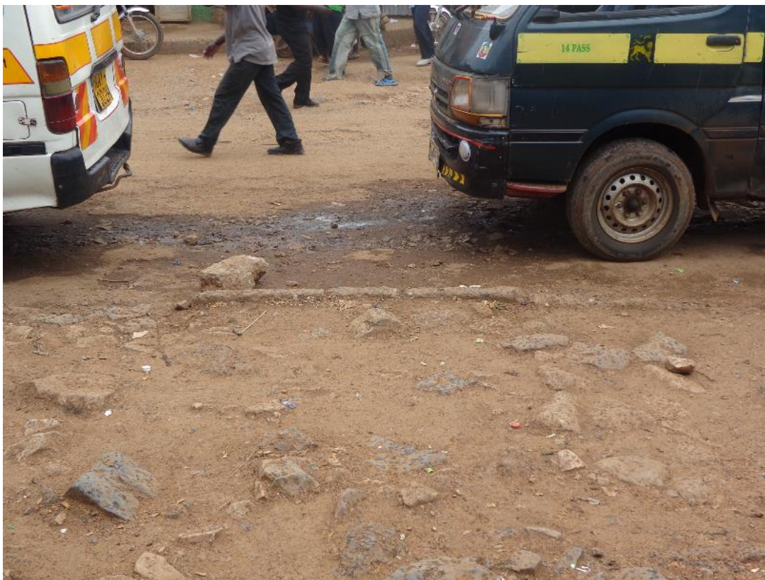
Plate 4.10: Eroded pavement in Kakamega Terminus
