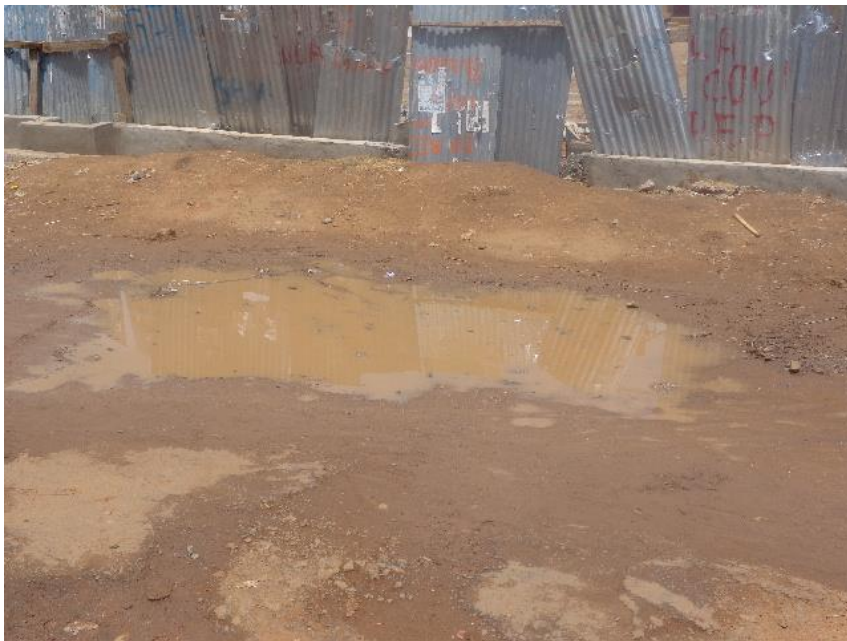
Plate 4.1: Drop Off Section Having Puddles of Water (Bungoma Terminus)
