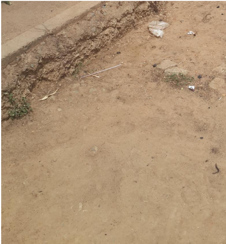
Plate 4.2: Eroded drop off next to kerb (Kendu Bay Terminus)
