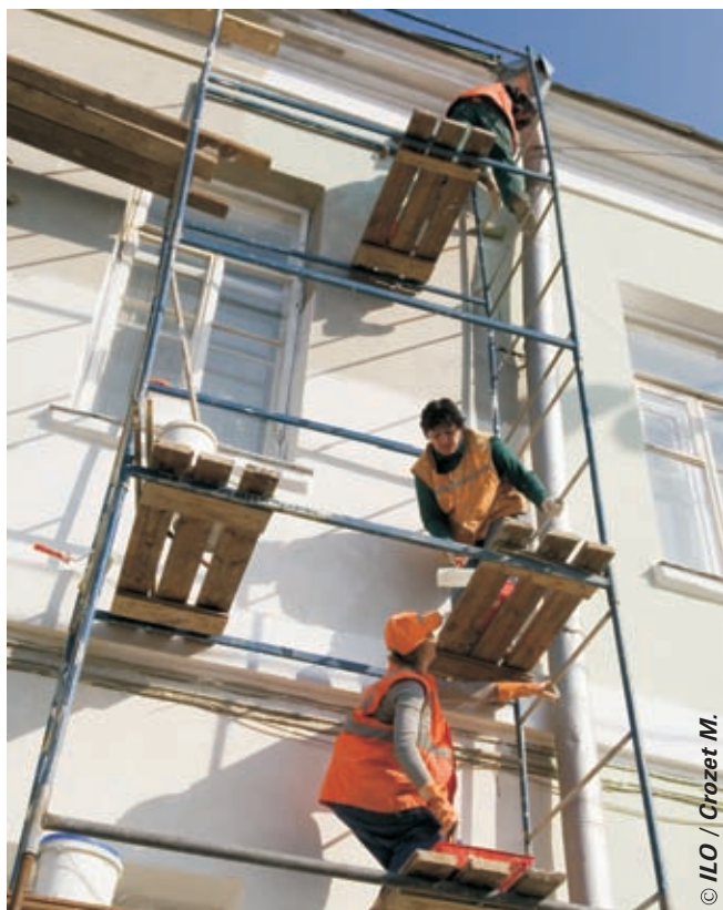
Building repairs at one of the central streets in Moscow (without proper security measures).
